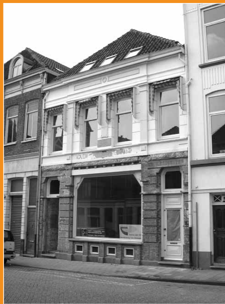
The house where Joris Ivens was born being renovated. © Photo Koos van Lith.
